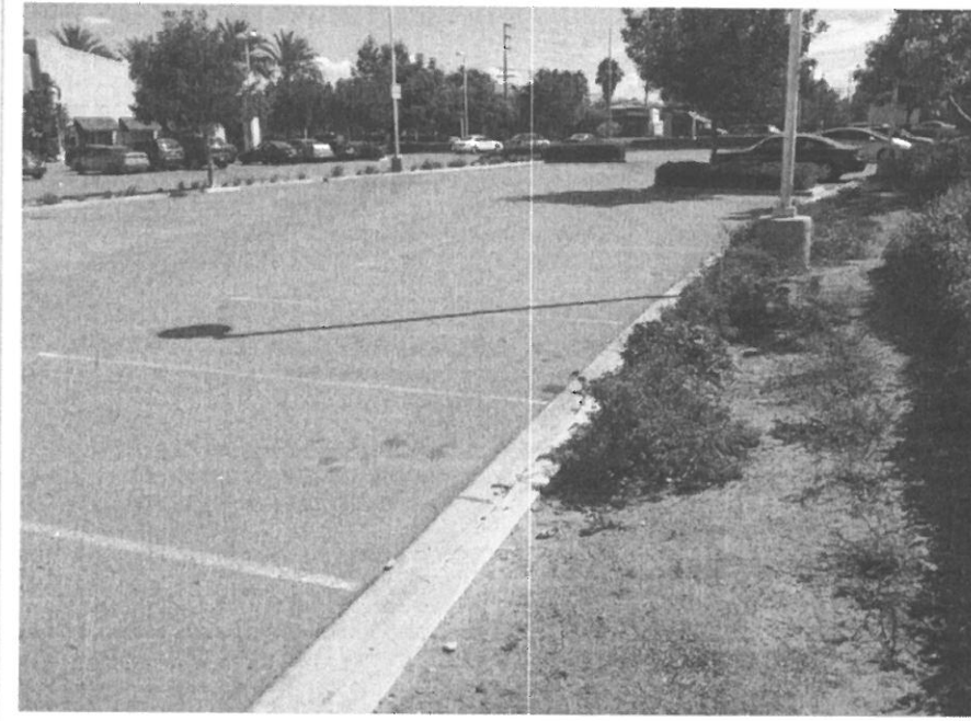
Area Missing Landscaping
