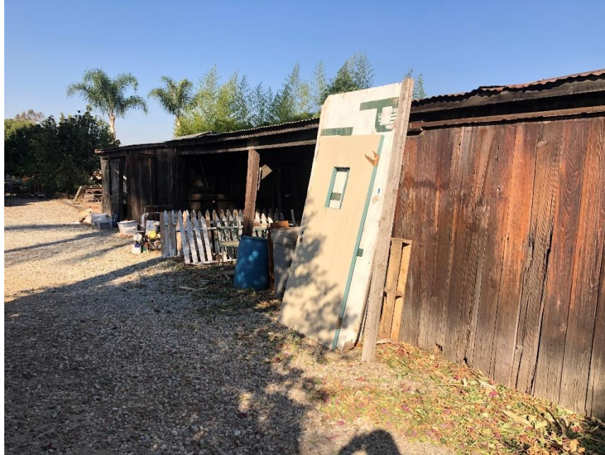
Figure 11A. Ancillary Building No.1 (view northwest), 2112 S. Oaks Avenue SOURCE: Sapphos Environmental, Inc., 2020
