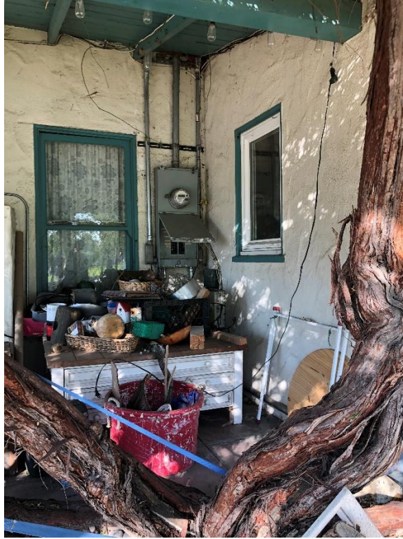
Figure 6B. Eastern Façade (view northwest), 2112 S. Oaks Avenue SOURCE: Sapphos Environmental, Inc., 2020
